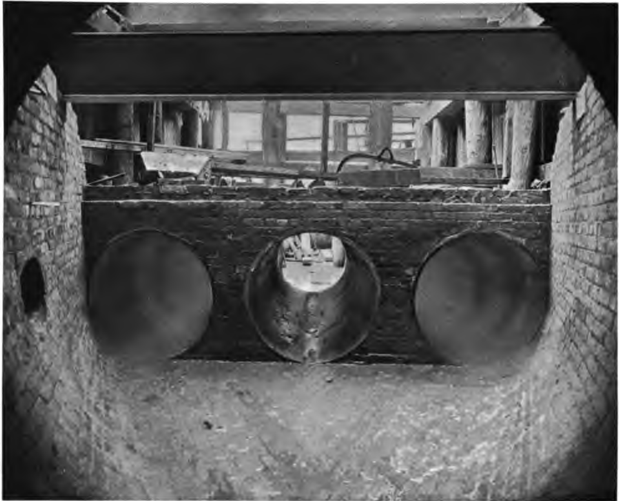
THREE PIPES SUBSTITUTED FOR LARGE BRICK SEWER AT 110TH STREET AND LENOX AVENUE
